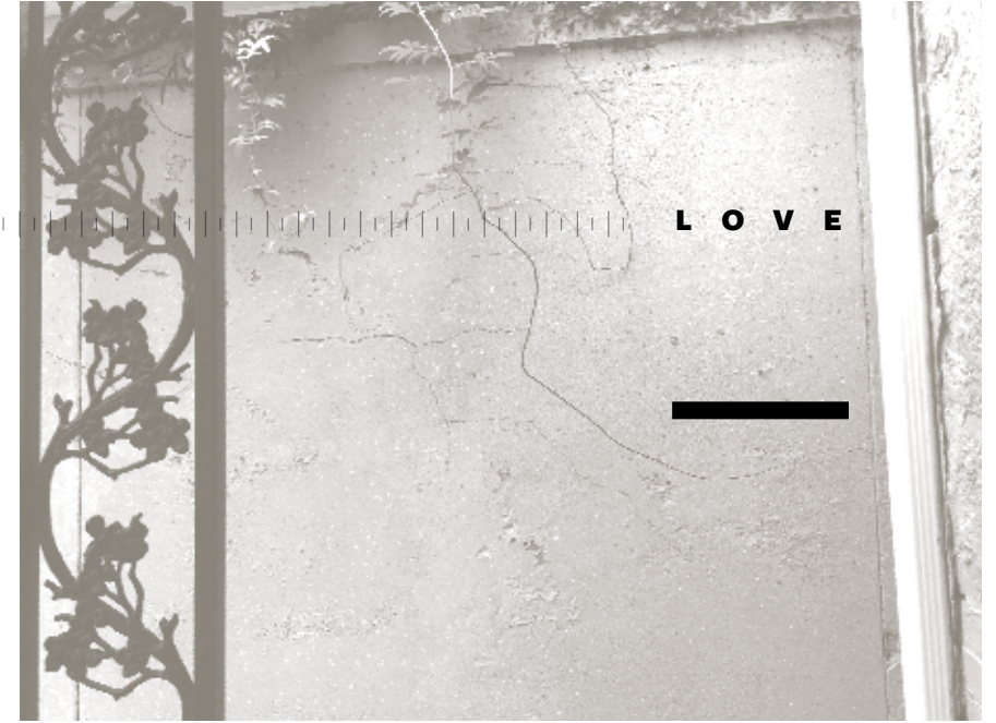
WALL CRACK MIMICS VINE | SAVANNAH, GEORGIA, 2015
